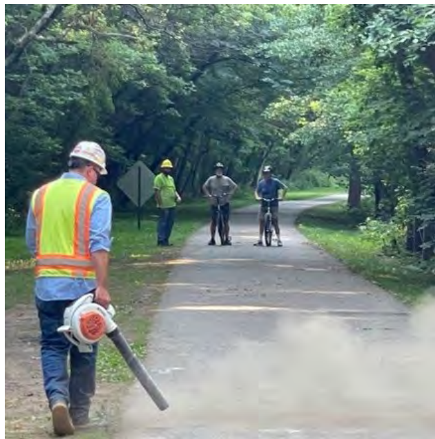
Figure 11: Permeable pavement must be frequently leaf blown or vacuumed to keep the voids between granules clear
