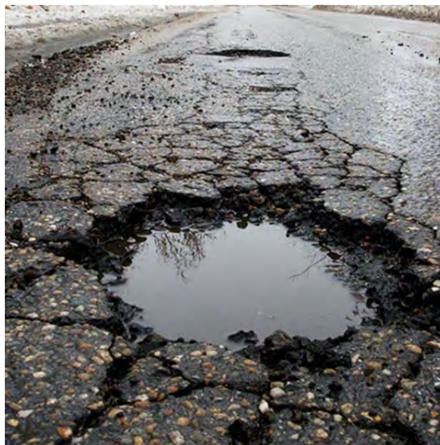
Figure 12: Asphalt cracks and creates potholes as a result of inundation and/or freeze-thaw cycles
