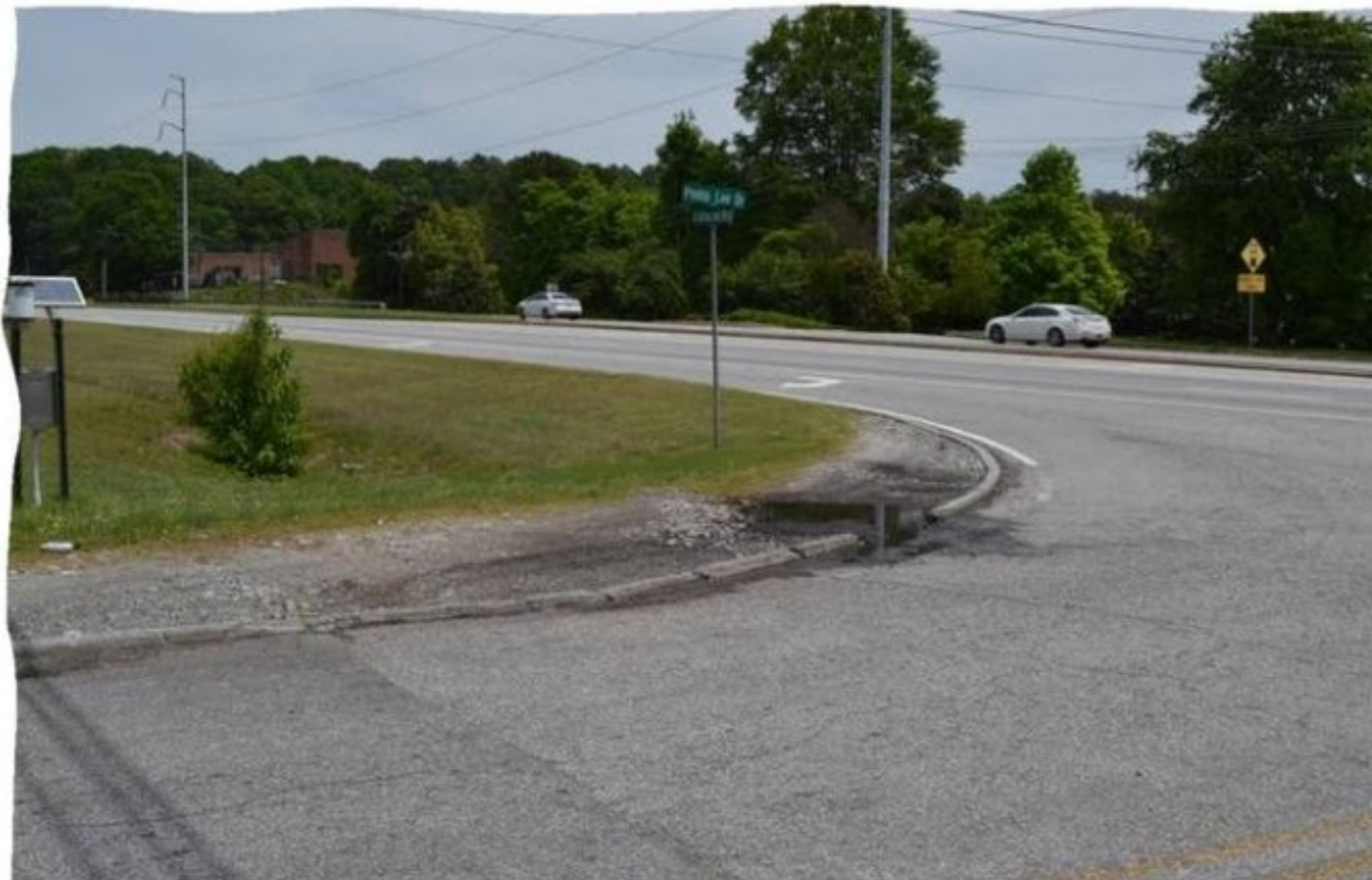
Example of Curb Cracking and Off-Road Rutting at Intersection of FIB & Phillip Lee Dr
